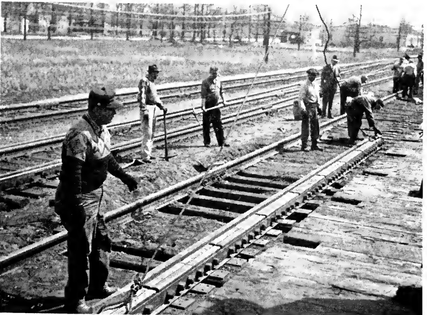
Fig. 3. Setting in Place the West Test Panel Before Renewing the Ties and Ballast
